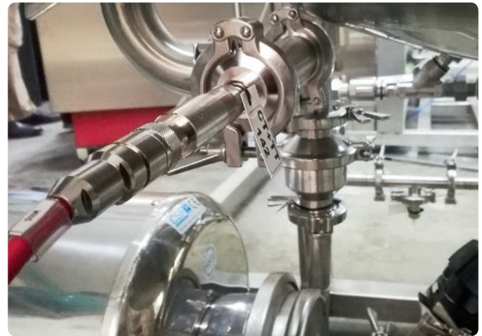
Figure 3: UPW conductivity measurement at the tank outlet after reverse osmosis.
